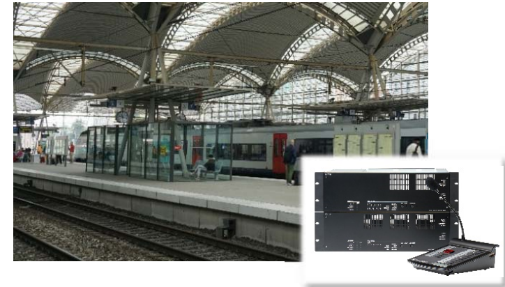
VX-3000 Series Voice Alarm System: Delivered to railroad stations in Brussels, Belgium
